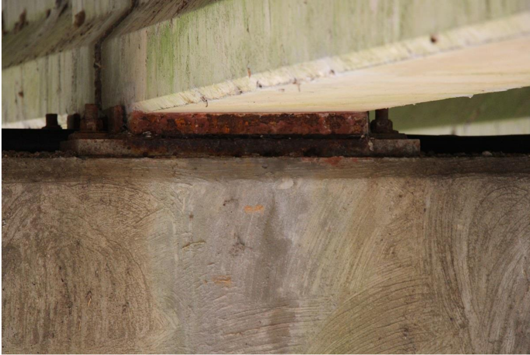
Condition Photo 30: Rusted steel bearing assembly, typical.
