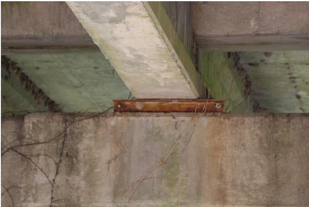
Condition Photo 31: Typical corroded bearing restriction device.
