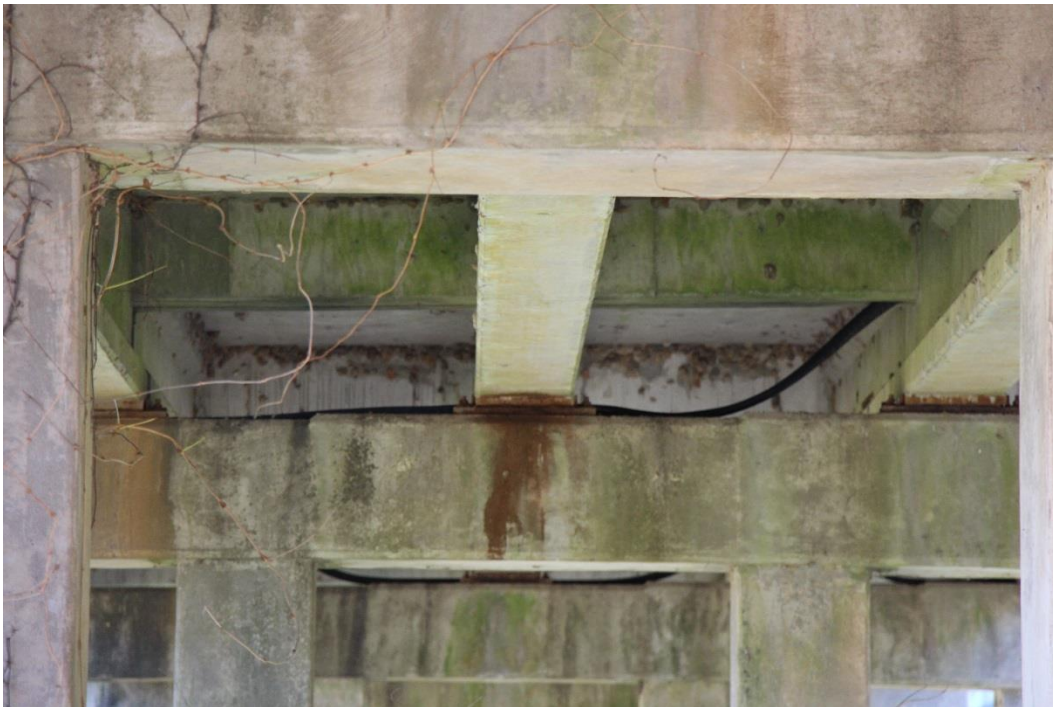
Condition Photo 29: Typical expansion joint failure.
