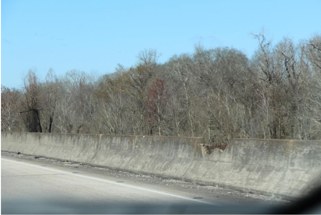
Condition Photo 20: North concrete barrier collision damage with exposed steel.
