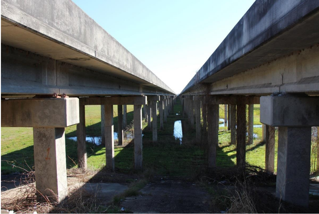
Character-defining Feature Photo 3: Detail of prestressed concrete girder superstructures (Recall No. 007300 on left and Recall No. 007310 on right).
