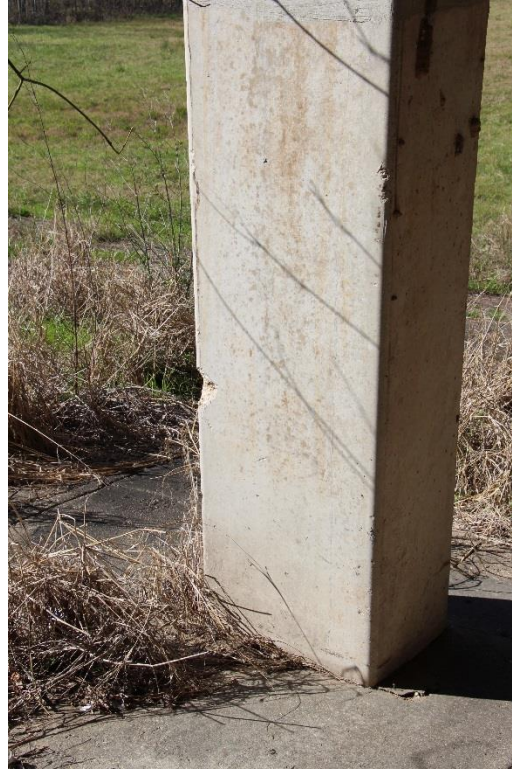
Condition Photo 12: Concrete spall on intermediate precast concrete bent pile.
