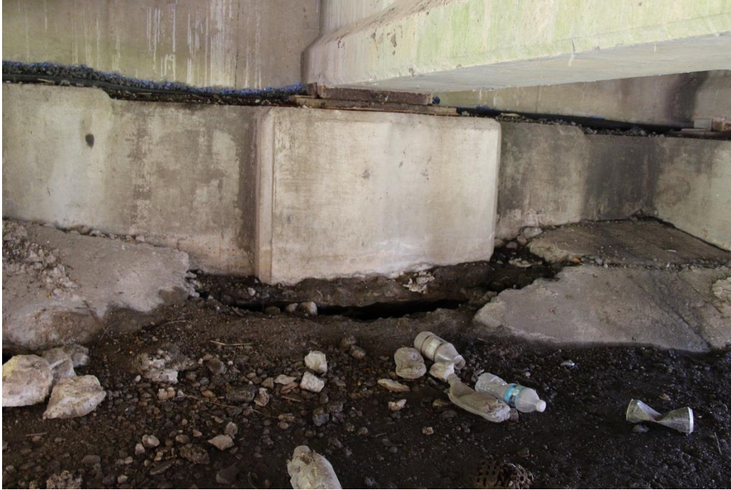
Condition Photo 24: Erosion and exposed bottom of end bent 1 and failed concrete slope protection.
