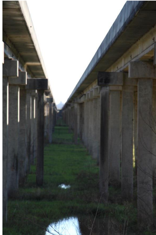
Condition Photo 6: Elevation of bents from between the two bridges showing the extension of the bents for both bridges.
