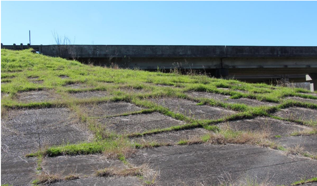
Condition Photo 22: Typical vegetation growth on the concrete slope protection.
