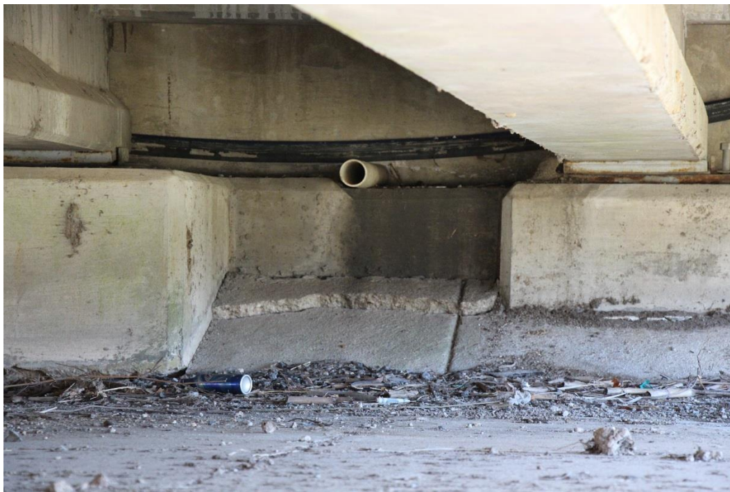
Condition Photo 13: Failed compression joint and failed concrete slope protection.
