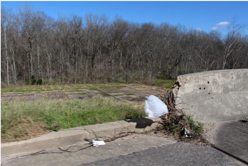
Condition Photo 21: Collision damage and exposed concrete on the barrier terminal wall.
