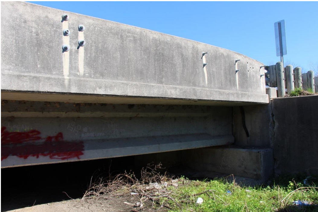
Condition Photo 27: Typical graffiti on the south exterior concrete beam, span 77.
