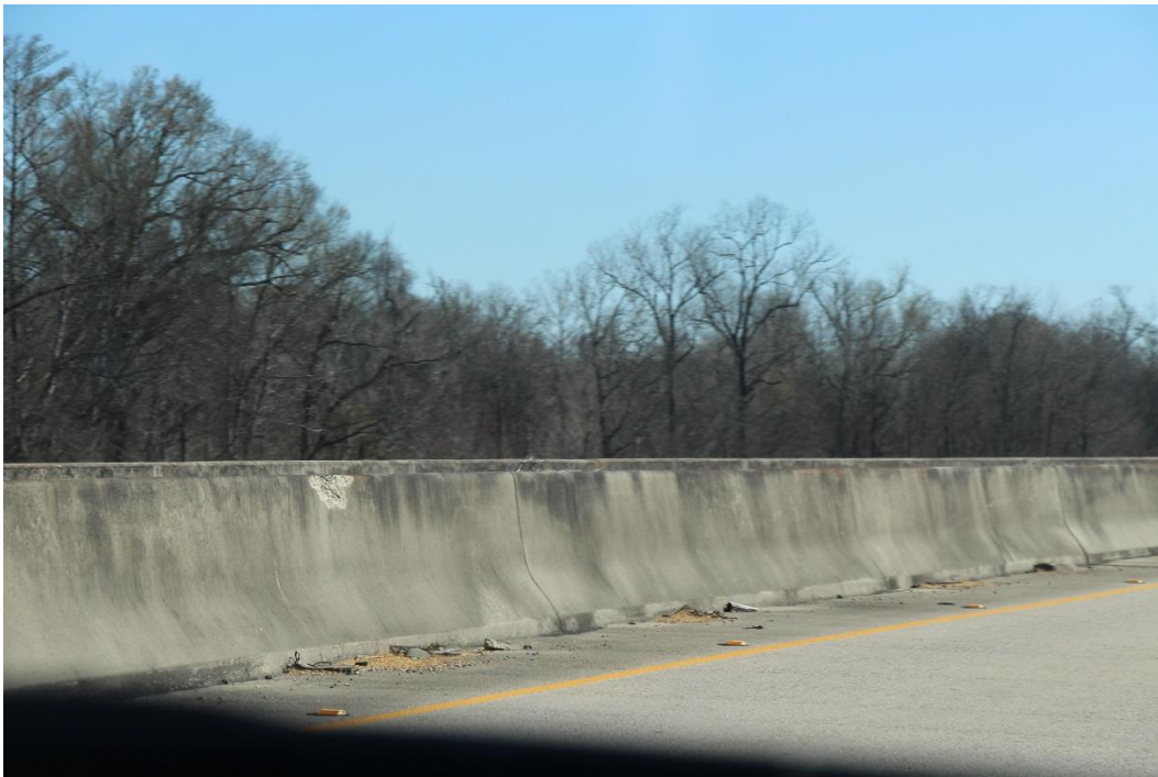
Condition Photo 5: Concrete spall on barrier and typical debris on shoulder.
