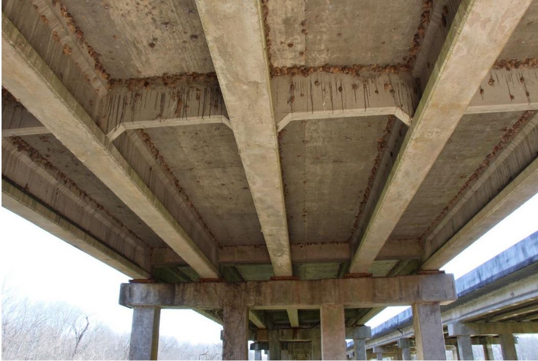
Condition Photo 26: Dirt dauber nests on the underside of the superstructure and cracking with efflorescence.
