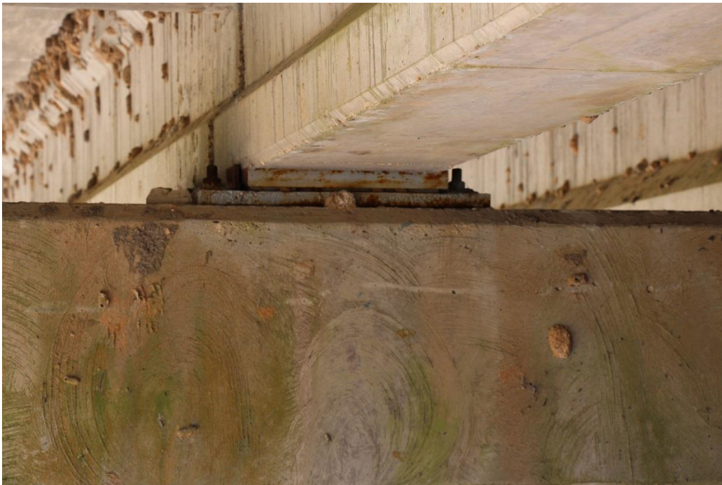
Condition Photo 15: Corrosion on the bearing assembly on the bents, typical.
