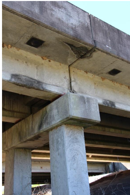
Condition Photo 19: Spall in concrete deck overhang.
