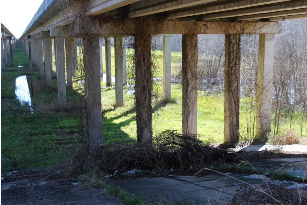
Condition Photo 8: Typical vegetation growth on the substructure units and part of the superstructure.
