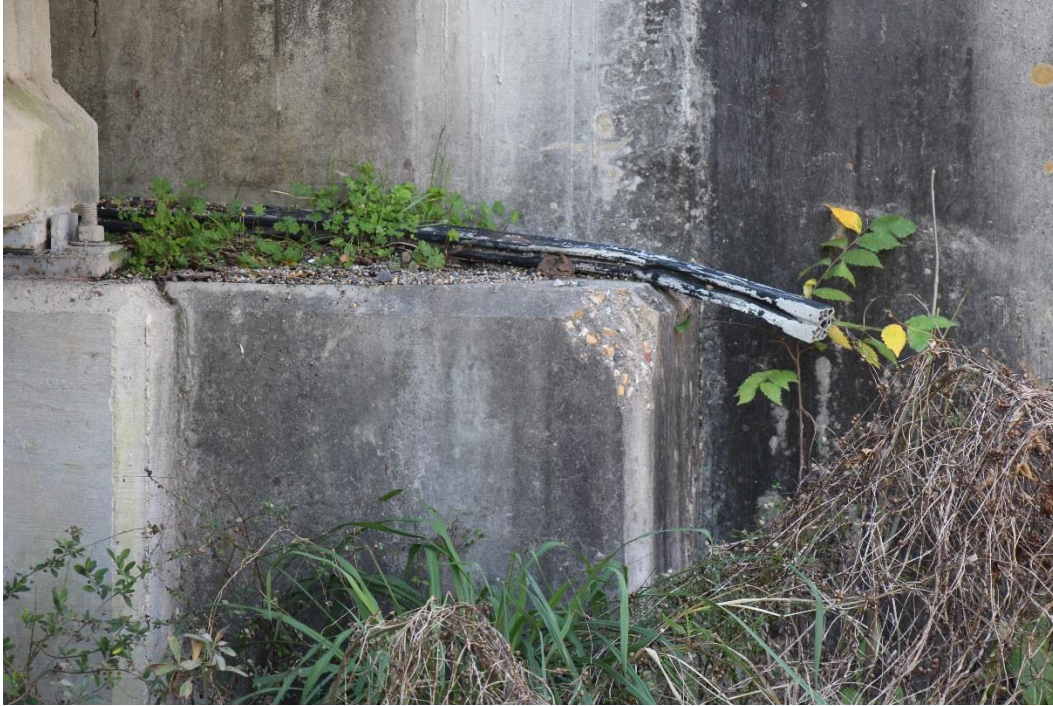
Condition Photo 10: Debris and vegetation on the end bent 1 seat and the failed compression seal strip.
