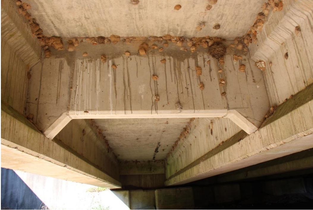
Condition Photo 28: Cracked concrete diaphragm between concrete beams, typical.
