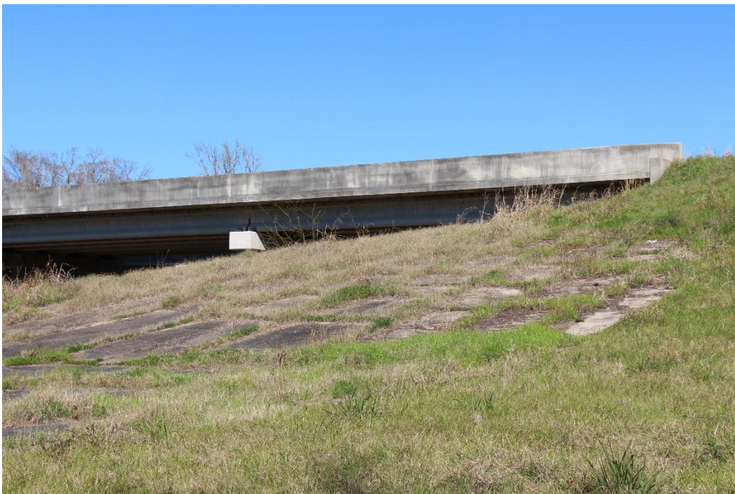
Condition Photo 7: Typical vegetation growth on the concrete slope protection.
