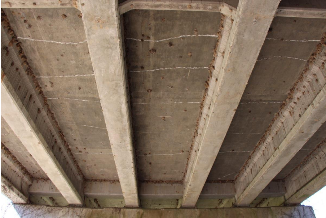
Condition Photo 14: Dirt dauber on the underside of the superstructure and cracking with efflorescence.
