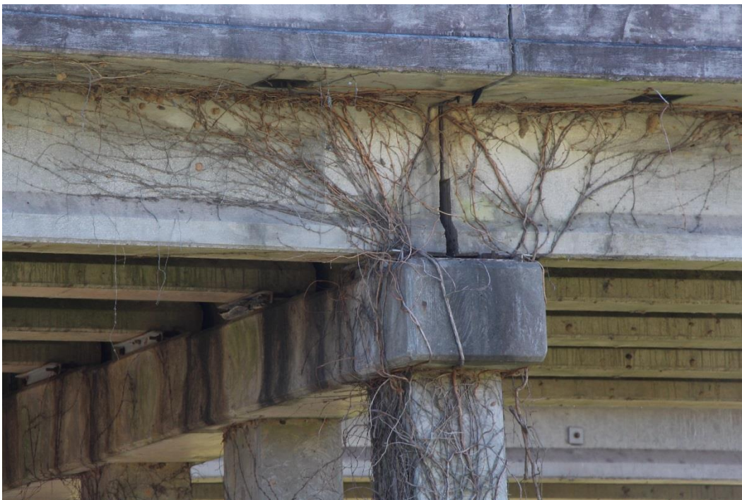
Condition Photo 23: Typical vegetation growth on the substructure units.
