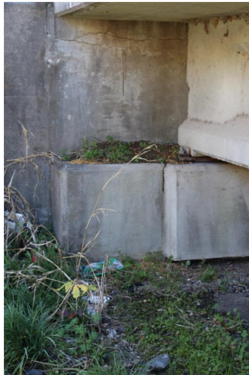
Condition Photo 11: Horizontal cracks on the end bent 78 backwall, dirt daubers on the concrete beams, and debris and vegetation on the beam seat.
