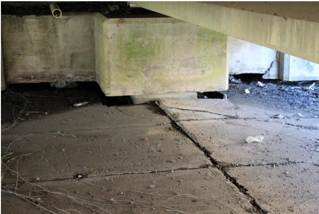
Condition Photo 9: Erosion and exposed precast concrete pile at end bent 1 and failed concrete slope protection.
