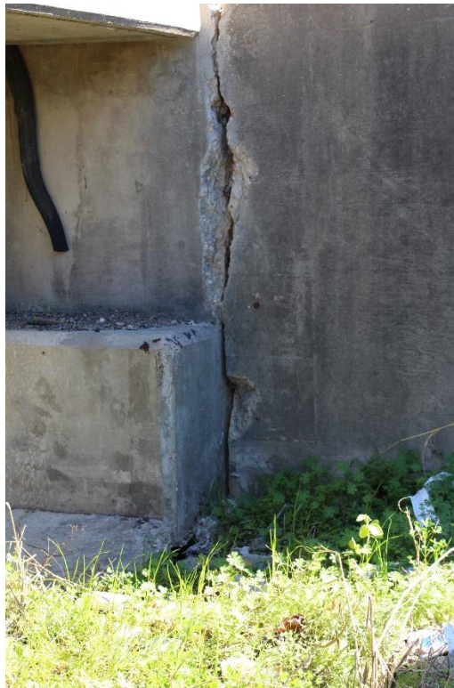
Condition Photo 25: Concrete spalled end bent 78 on the south side.
